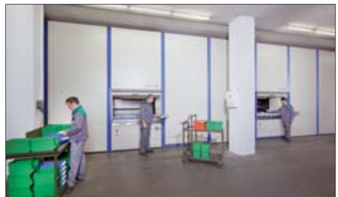
Two Hänel Multi-Space® units, each almost 393.10' wide, constitute the central store for the production hall
